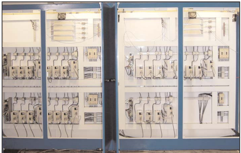
Control cabinet with Mitsubishi C64 CNC Controllers
