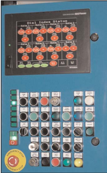
Front of one of the operator control panels
