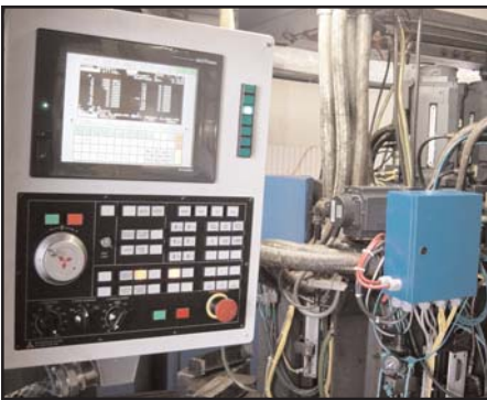
Closer view of the Operator Interface
