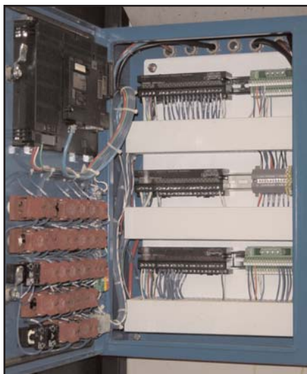
Inside of the operator panel with CC-Link Remote I/O modules enabling considerable reduction of wiring
