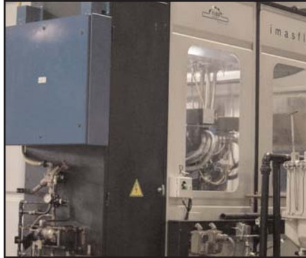
Black cabinet contains the pneumatic valve manifolds. Blue cabinet contains the CC-Link Remote I/O modules that control the valve manifolds. Wiring distances are minimized.
